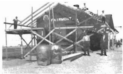
Repairs to Fairmont, Okla., Station after recent cyclone. M. Larkin, Agent, and W. C. Fisher, Foreman B & B in foreground.
